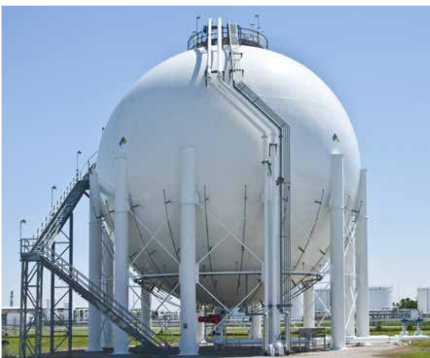
A sphere specialty vessel with a diameter of 76 feet, fully completed and painted. Image courtesy of Matrix PDM Engineering
