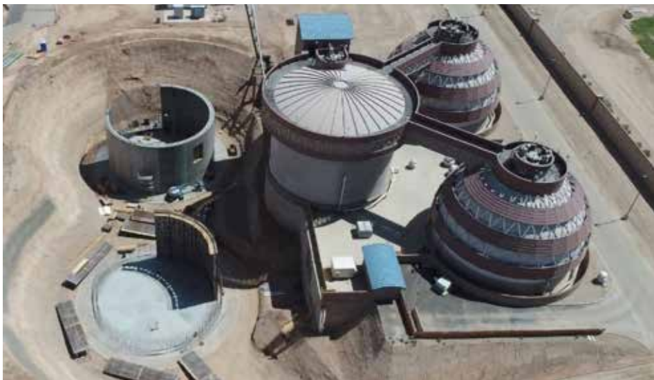
Anaerobic egg-shaped digesters. Two digesters are completed, and two additional are being built. Image courtesy of Matrix PDM Engineering
